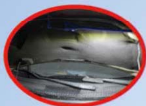
Engine room lighting
